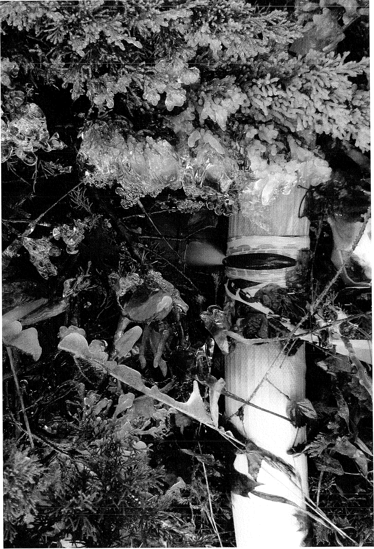
FIRE LINE AT 4 LAUREL AVE. LEAKING 12-06-10
